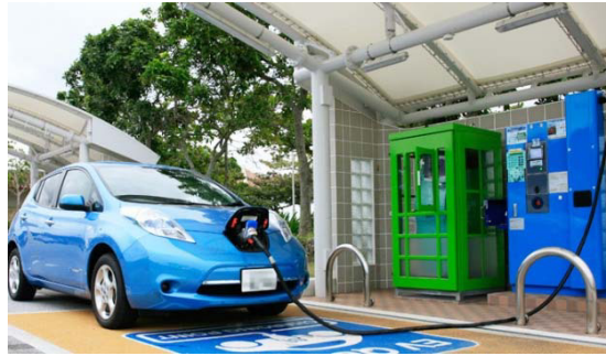
Figure 12: Charger station for EV car
