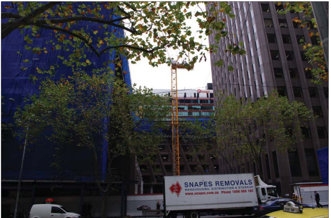
1466. The St James AMP Centre now fills the site with continued redevelopment
