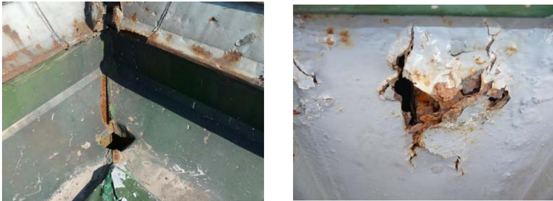
Fig. 4 Deterioration of the roof (left: corrosion of the metal at the junction of the roof and gutter; right: cracks in roof)
