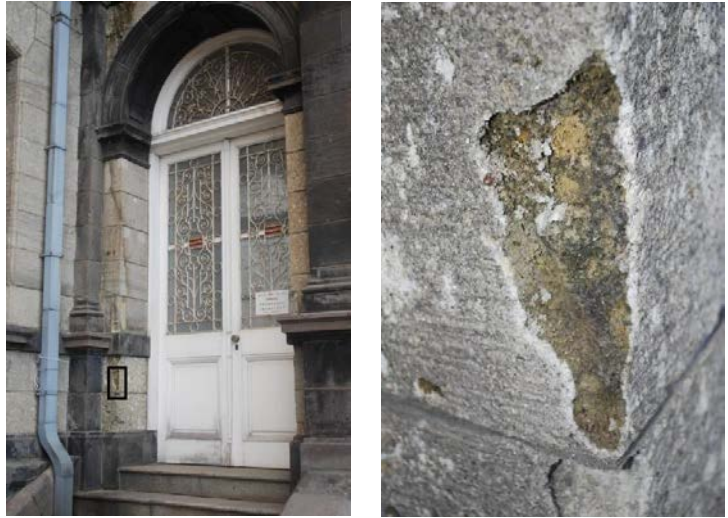
Fig. 3 Deterioration of stone wall surface (right: enlarged image)
