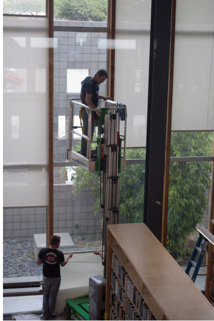
Workers applying UV-filtering film on the Poetry Center's big bank of windows. Photo by Sarah Kortemeier.
