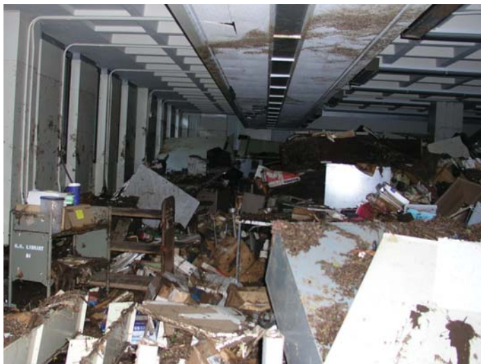
Hamilton Library's acquisitions department, shown here, is where the water first rushed in, hitting the ten-foot-high ceiling.
