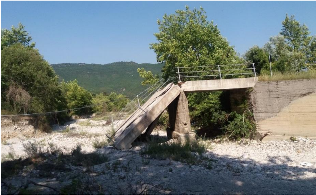
Photo No. 2 – The collapsed bridge that is located outside of the village.
