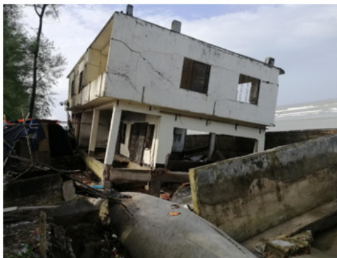
Figure 1: Building damage near to Himchari
