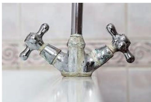
Figure 5: Lime scale on a water tap
