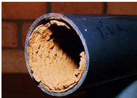
Figure 3: Limescale in pipes
