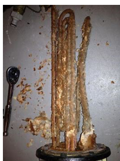
Figure 4: Lime scale on boiler heaters
