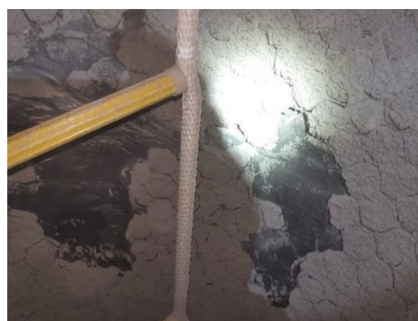
Figure 11. Wall wear of cyclone separator
