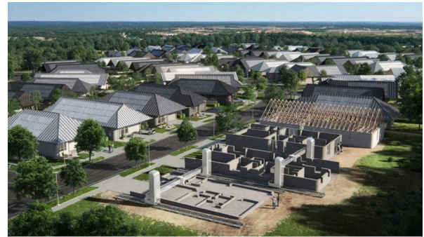
Figure 3. The world's largest automated 3D building project is being implemented in Georgetown, USA
