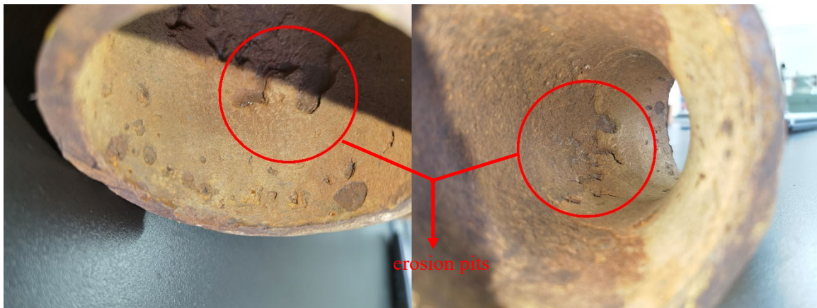
Figure 2. Erosion pits inside the vent pipe elbow
