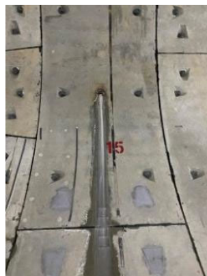
(b) Leakage of grouting holes
