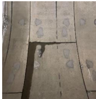
(a) Leakage in the longitudinal seam
