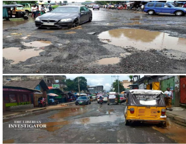
Figure 9. Potholes on the roadways of Monrovia [25]
