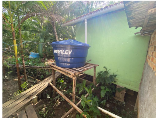
(B). Front view of the secondary tank.
