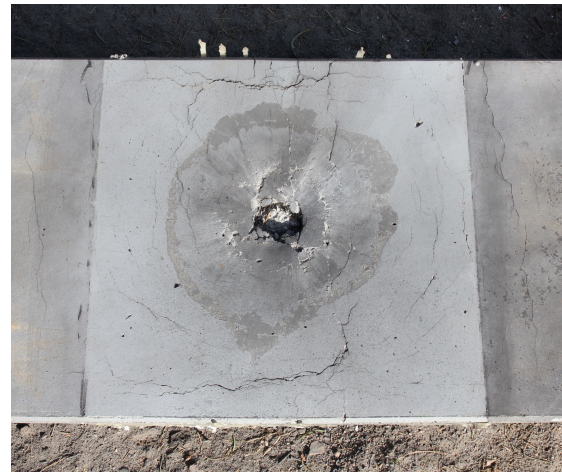
FIGURE 10. Blast damage on the impacted side of an HPFRC panel with PU coating on both sides.
