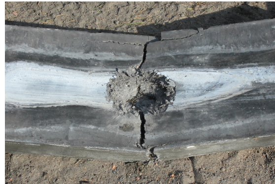
FIGURE 13. Complete failure of a bare HPFRC panel due to blast; rear side.
