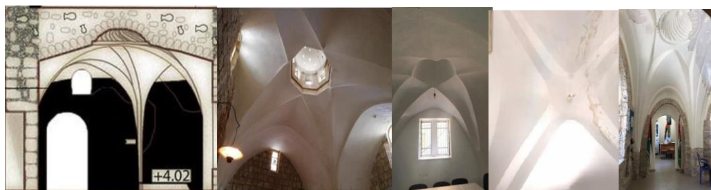
Figure.6: Photos represent construction examples of fan vaulting (drawing and photos taken by the author, 2022)
