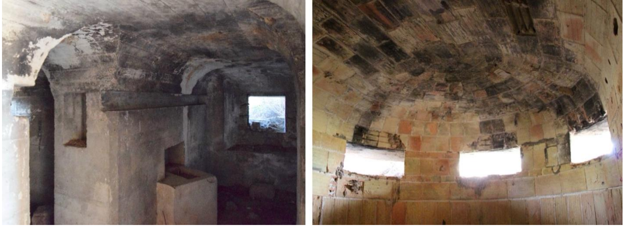
Figure 8: Left: the interior of a reinforced concrete bunker used in Arborea, Italy; right: the interior of a bunker with a brick formwork in Balsares, Spain (photos by A. Martínez-Medina).
