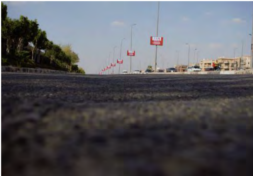
Fig. 26: Pavement damage. (Source: the authors)
