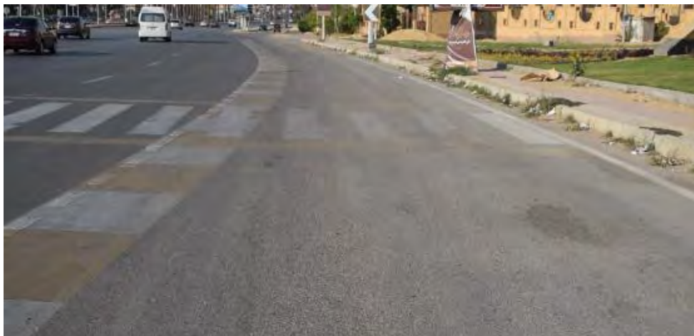
Fig. 27: Absence of special rain drainage. (Source: the authors)
