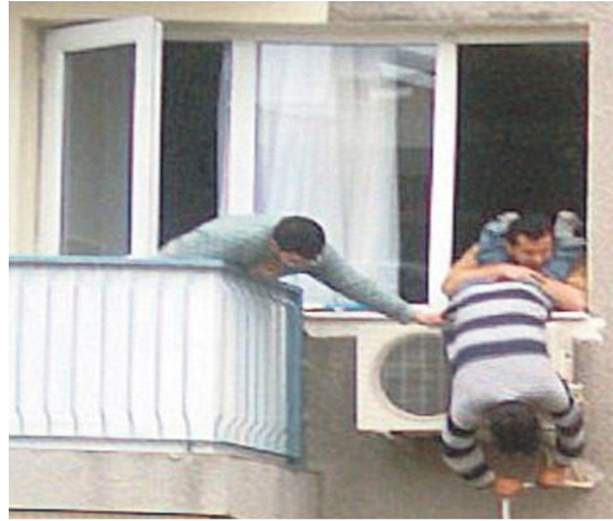
Figure 3. Air conditioner technicians risking lives to install units. (Source: Online Mail Newspaper, 24 Octobe,2008)
