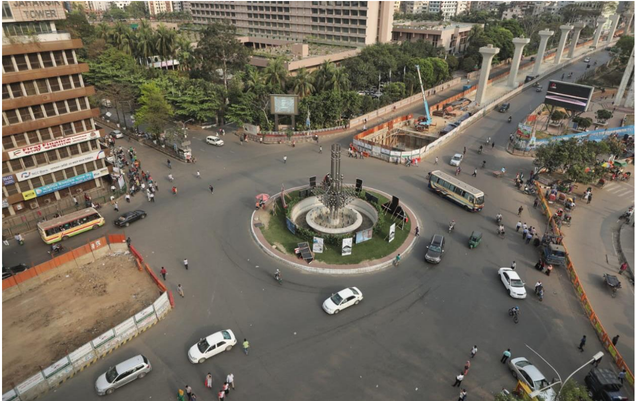
Figure 2: New modes of transport being added in Dhaka. The photo shows the ongoing construction work of elevated MRT at the Karwan Bajar node. Image courtesy: Dhaka Tribune
