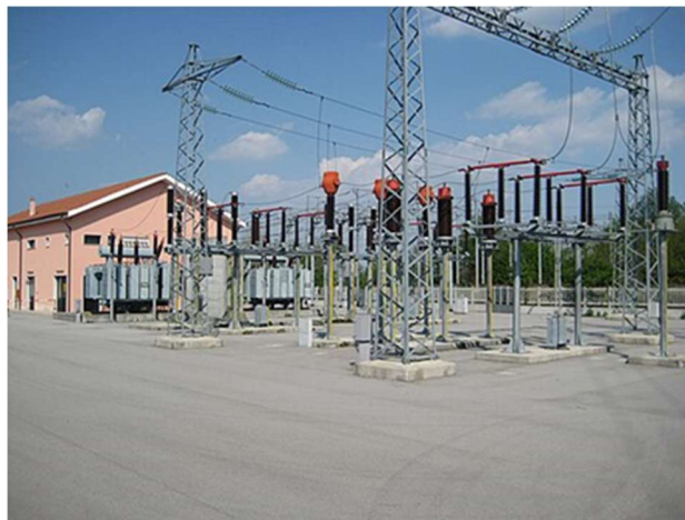
Figure 1. Example of a railway electrical substation
