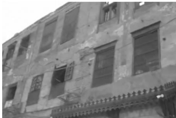
Figure 5. Deterioration in the elevation of Wikālīṭ al-'Anbariyin . (Source: Dardasha Tareq, 2019. https://www.youtube.com/watch?v=-ZtLLsrwJU8 )
