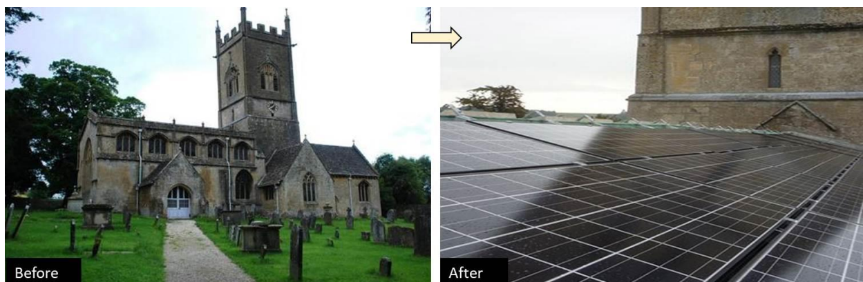
Figure 11: International attempt 2; thermal retrofit for improving the St. Michael and all Angels Church in Withington, England (Author & participant students)
