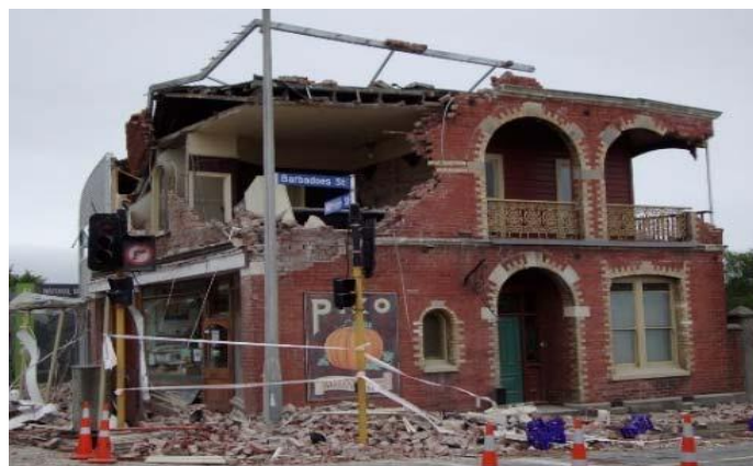
Figure 8: URM Building on Barbados St. Damaged after the Earthquake (Schwede66 2011)
