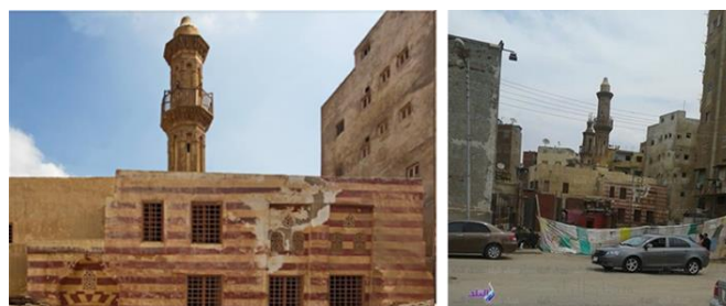
Figure 12: shows the effect of low maintenance for the mosque.
