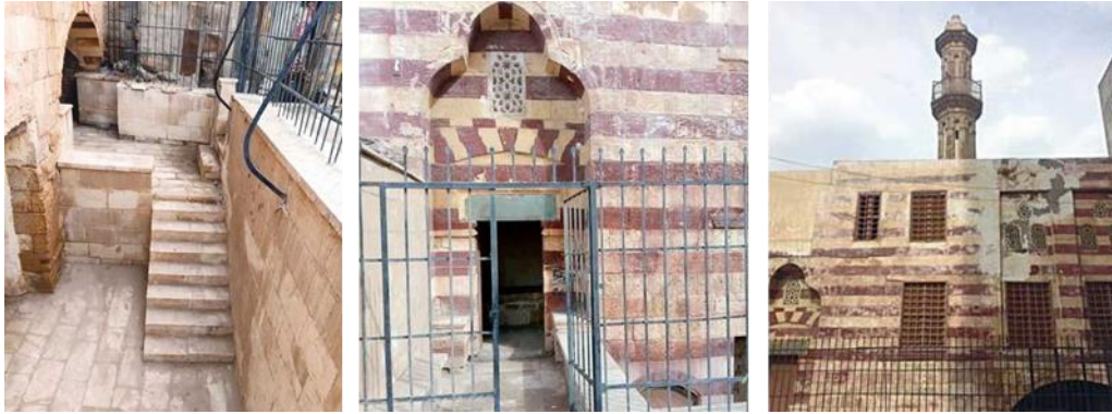
Figure 6: shows the entrance and the shape of el Amir Hamad mosque and minaret, and the rate of deterioration
