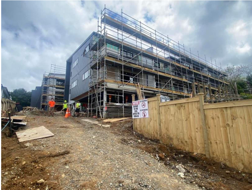
Figure 6. Case Study B: 23 walk-ups in Ellerslie, Auckland Central (under construction) (Authors' photo, 2021)
