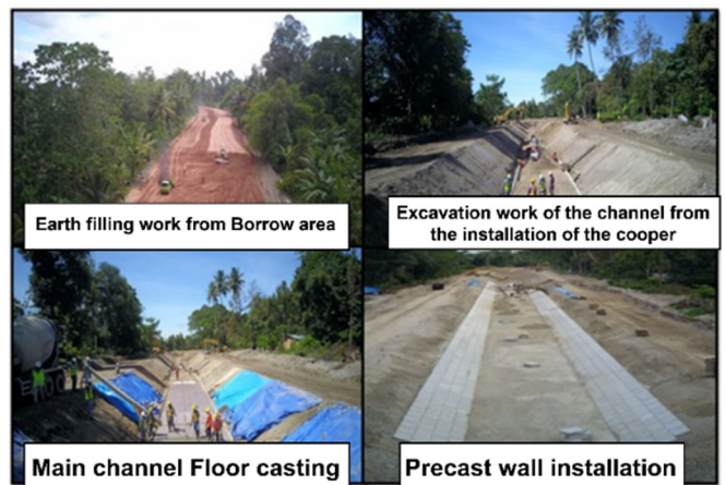
Fig. 6. Construction of the Baliase main channel on the right side after the design was reviewed.
