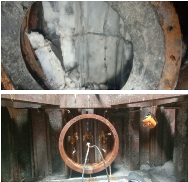
Fig. 15. The soil did not collapse after being injected at the entrance hole in the pit of the construction area.
