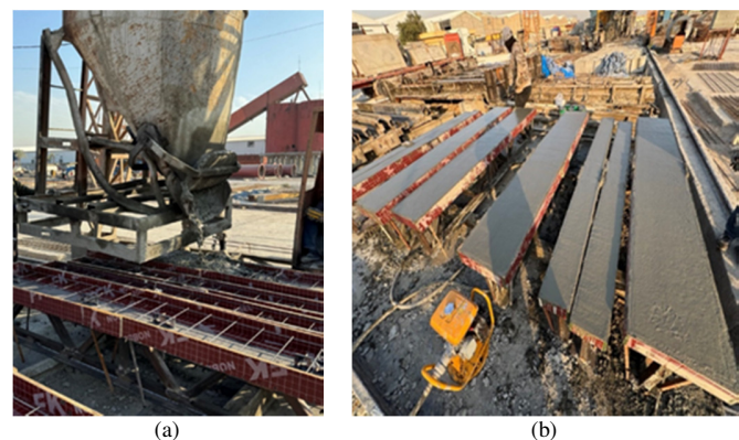
Fig. 7. Steps of concrete pouring for SCTG and DCTG: (a) pouring stage of the concrete mix, (b) final stage after casting the top and bottom concrete deck slabs.
