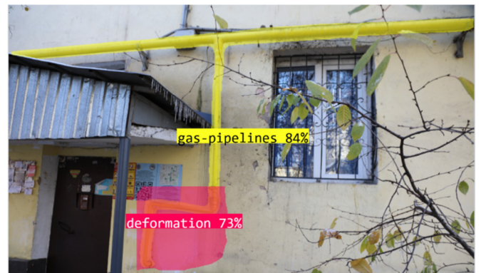
Fig. 4. Example of automatic deformation detection on outdoor gas pipelines using trained models.
