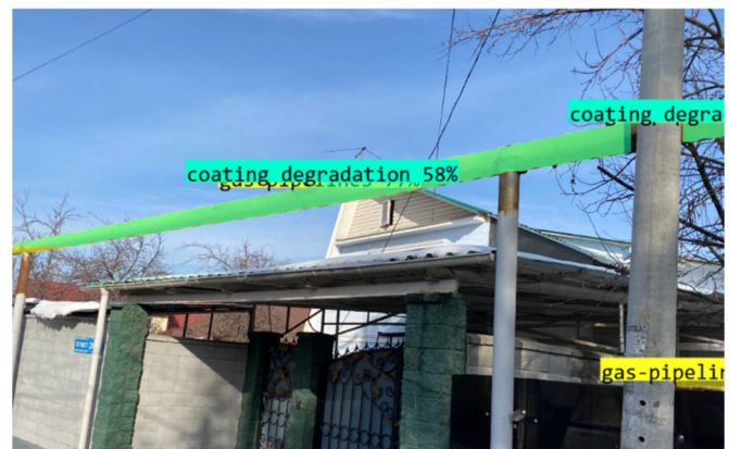
Fig. 5. Example of automatic coating damage detection on outdoor gas pipelines using trained models.
