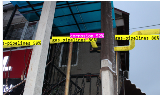
Fig. 3. Example of corrosion detection and gas network elements in a closed space using trained models.
