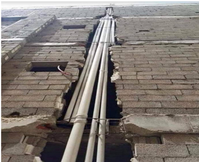
Fig. 1. Incorrect extension of sewer pipes in a commercial building.
