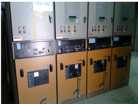
Fig. 2. Cell from the electric power system.
