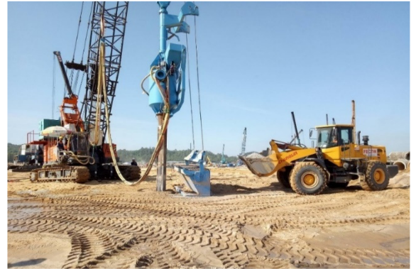
Fig. 1. Dry bottom feed stone column operation at the Long Son Petrochemical Project.
