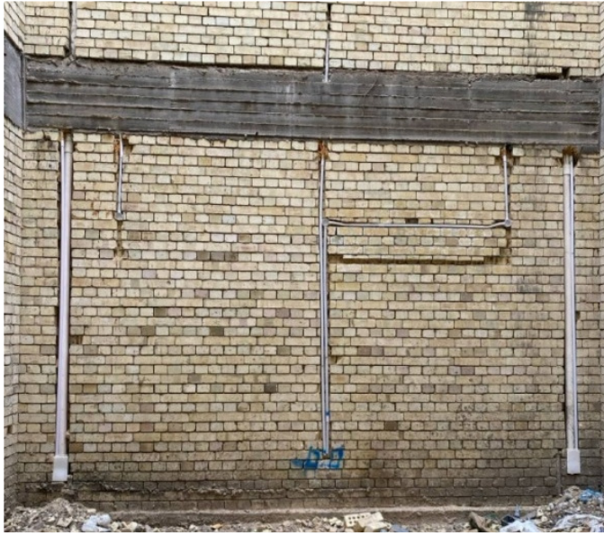
Fig. 1. Various service pipes passing through RC beams in commercial buildings.
