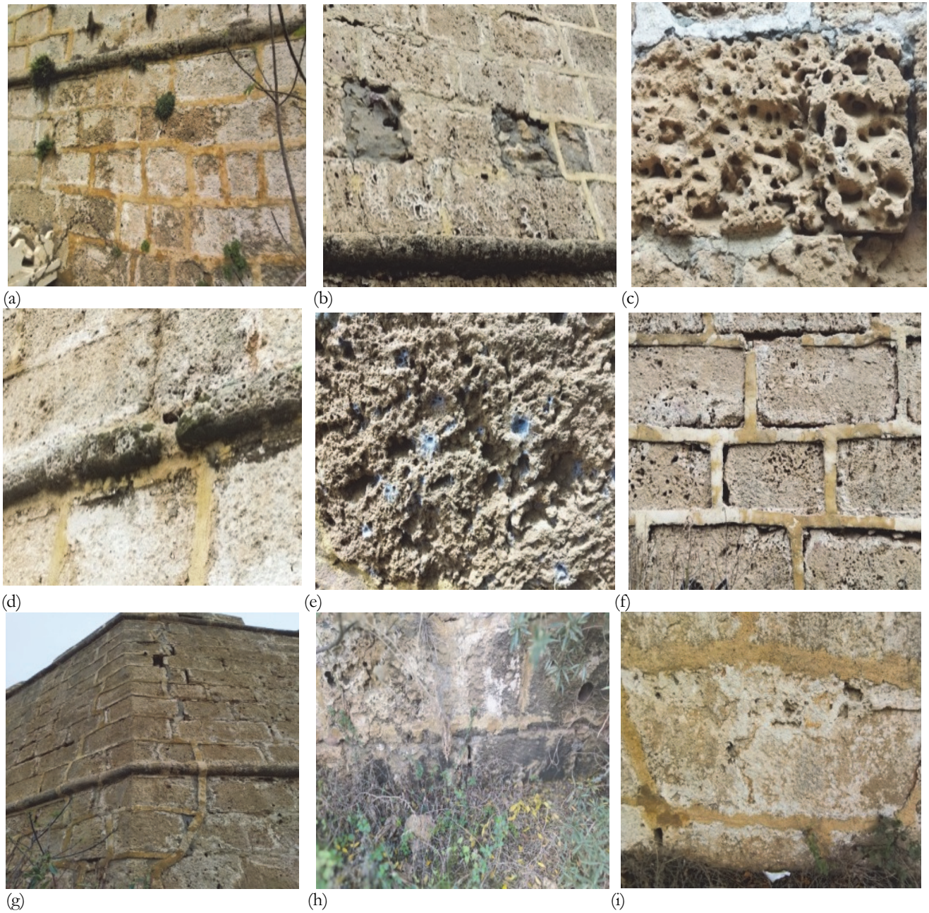
Figure 26: Southern fort façade type of damage (a) biological colonization, (b) scaling, (c) alveolization, (d) disaggregation and lichen colonization, (e) special biological colonization by a spider web, (f) erosion, (g)cracking, (h) black crust ,(i) effloresce.
