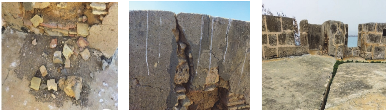
Figure 3: Damaged masonry walls on the terrace where the stone block samples were taken.
