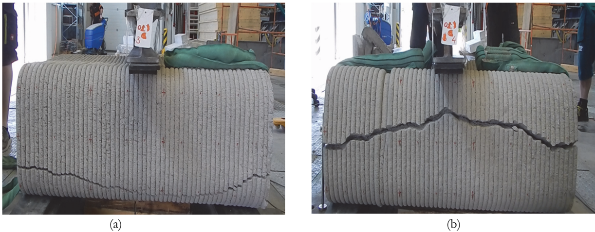
Figure 4: a) Fractured specimen CP18-03; b) Fractured specimen CP18-04.
