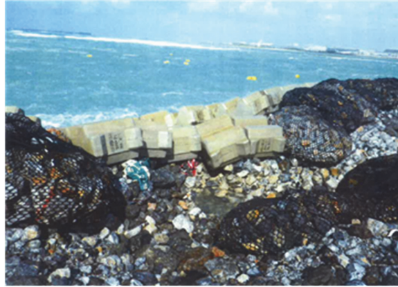
Photo 1 Damage of filter units due to high waves
