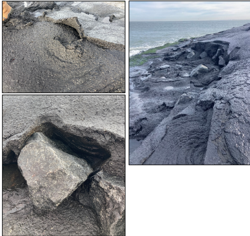
Figure 12. Photo of the erosion of the protection layer in 2023. Upward left: stage 1 - peeling of asphalt, downward left: stage 2 - pulled out stones, right: stage 3 – stones and asphalt are washed away.
