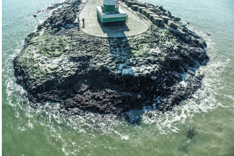
Figure 10. Photo of damage at the roundhead of the southern breakwater in 2022.
