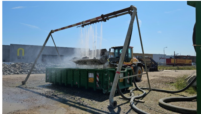
Figure 18. Set up for washing of stones which removed dust from the armour stone.
