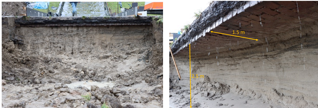
Figure 14. Start of cliff erosion at the asphalt road (left). Undermining 1.5 m after 5 hours of testing (right) and the erosion was almost terminated.
