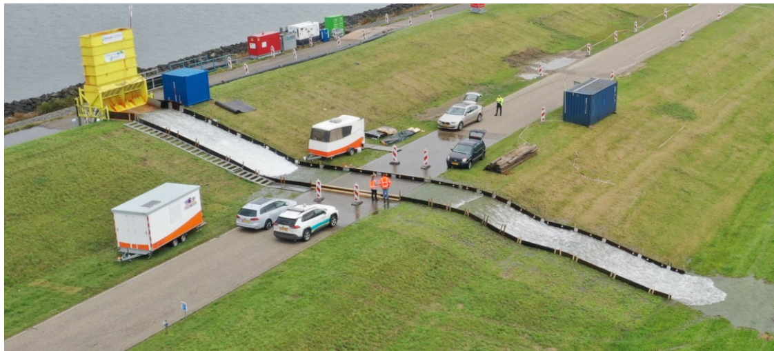
Figure 7. Test set-up at the dike with a wide berm and an asphalt road 3 m below the crest.
