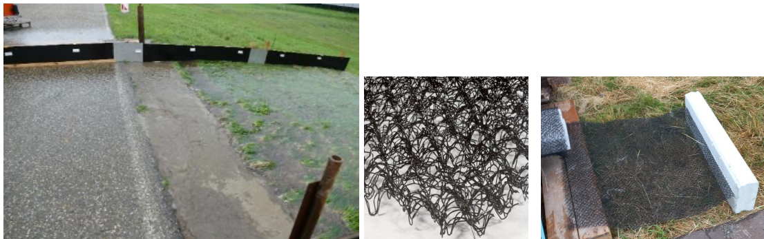
Figure 4. A block of Mixed-in-place of 0.6 m by 0.8 m to prevent failure at this transition (left). A concrete block with geogrid connected to give the grass a stronger connection (middle and right).
