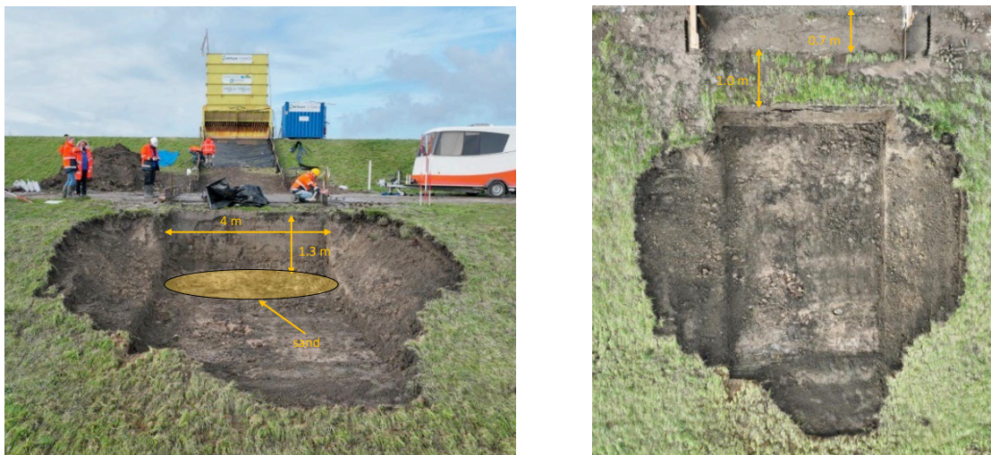
Figure 12. Creation of a cliff behind the asphalt road onto the sand core (left). Top view of the cliff erosion hole with the remains of 1 m grass cover with boulder clay underlayer and the 0.7 m wide Mixed-in-place block against the asphalt road (right).
