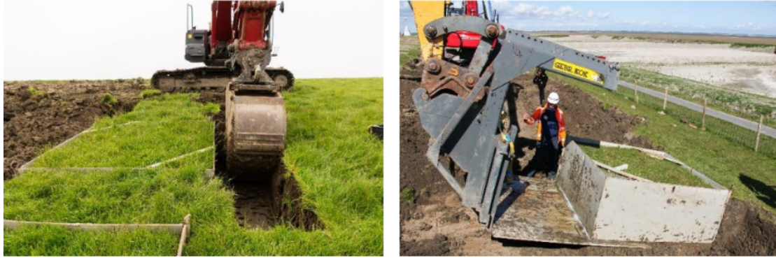
Figure 5 Excavation of the steel frame and pushing the bottom plate underneath the frame.
