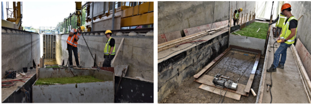
Figure 6 Removal of the side wall and the bottom plate in the Delta flume
