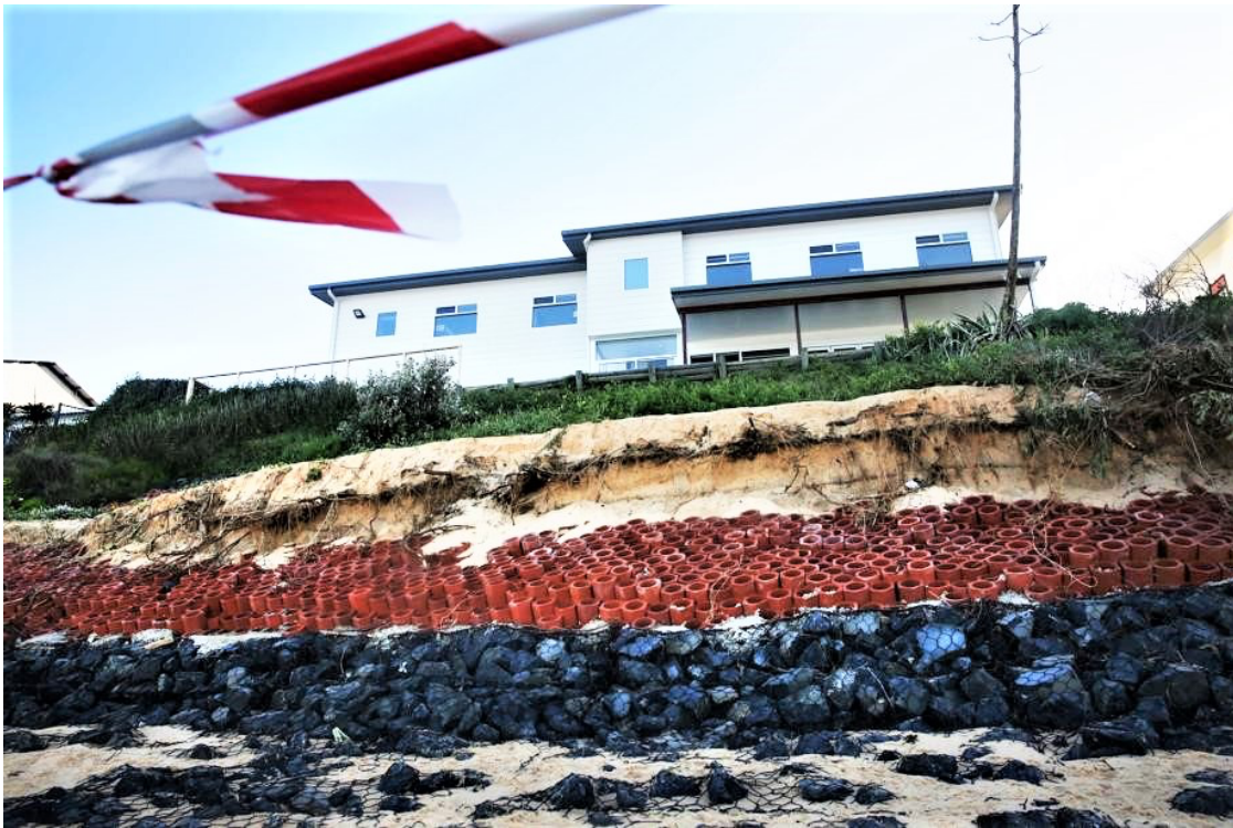
Figure 3. June 2016: a rare survivor of the storm: performed as expected, but failed by scour & sliding in 2020.
