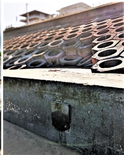
Figure 13. Loss of fill through gaps leads to loss of fill below the filter cloth.
