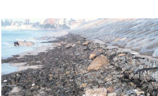
Figure 10. 1986 – Damage in first months of service
