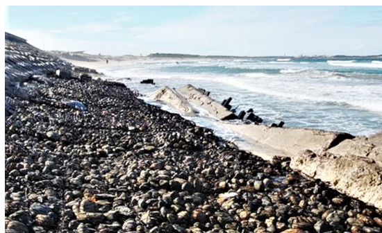
Figure 11 2007 Damage at the downdrift end
