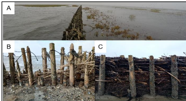
Figure 1 - Flooded brushwood groyne field with pioneer salt marsh vegetation on the island of Pellworm (A). Empty groynes at the field site (B) and refilled groynes with brushwood (C) after maintenance.
