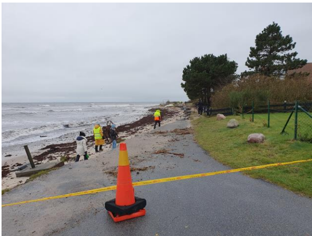
Figure 4 - Complete destruction of a road caused storm erosion. This part of the coast that has been subject to long-term coastline retreat.
