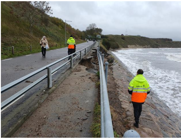
Figure 3 - Undermining of road caused by wave runup on a road bank protected by a revetment.
