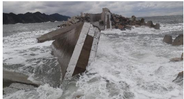
Figure 2 - Failure of the main breakwater at Section 2-2.
