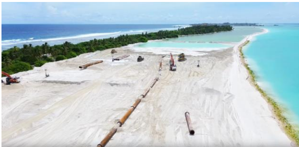
Figure 1 - Reclamation works and beach development at Hithadhoo Zone 2 in Addu City, the Maldives
