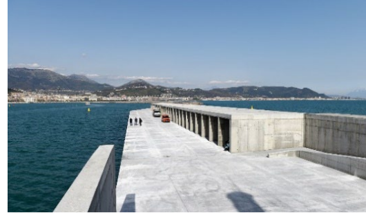
Figure 4. Final stage of the realization of the U-OWC breakwater in the Salerno's port.
