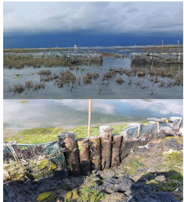
Figure 1 – June 2023, opening interventions. Top: removal of geotextile and poles. Bottom: removal of geotextile only.
