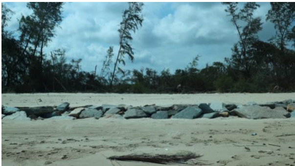
Figure 1 - The revetments at Pak Phanang beach drowned under the sand deposition, leading to question their capability to protect the coasts in extreme conditions.
