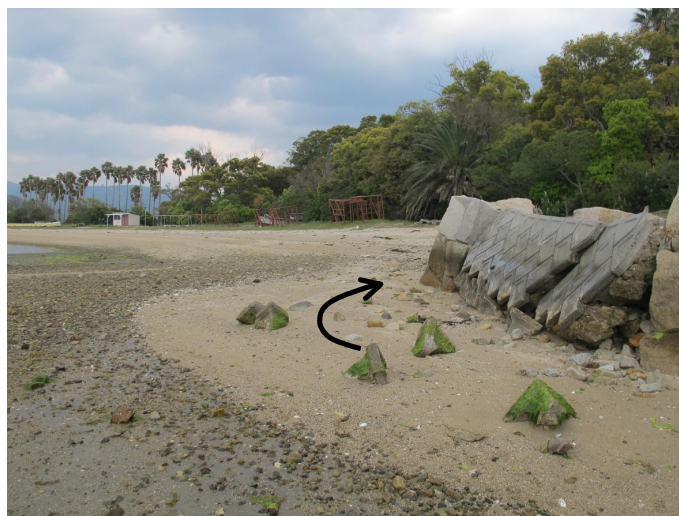
Figure 13. High water marks showing longshore sand transport turning around damaged seawall.
