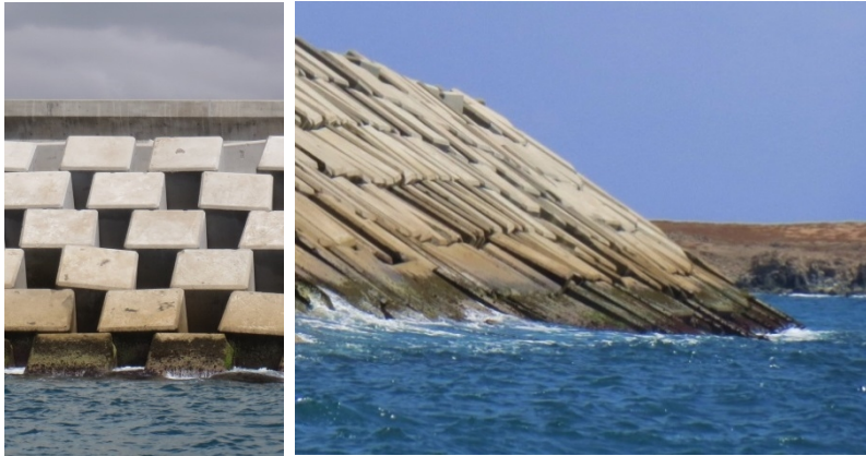
Figure 6 Picture of a breakwater with a single-layer of Cubes ( i.e. a lower roughness of the armour layer).
