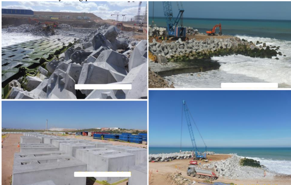
Figure 16. Pictures showing the construction and placement of the blocks along the breakwater root
